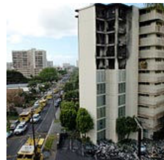
Five apartments were left blackened shells by the fire, and debris rained down on the parking lot below, damaging a car. The building is one of many on O'ahu built before 1975, and therefore not required to have an automatic sprinkler system.
